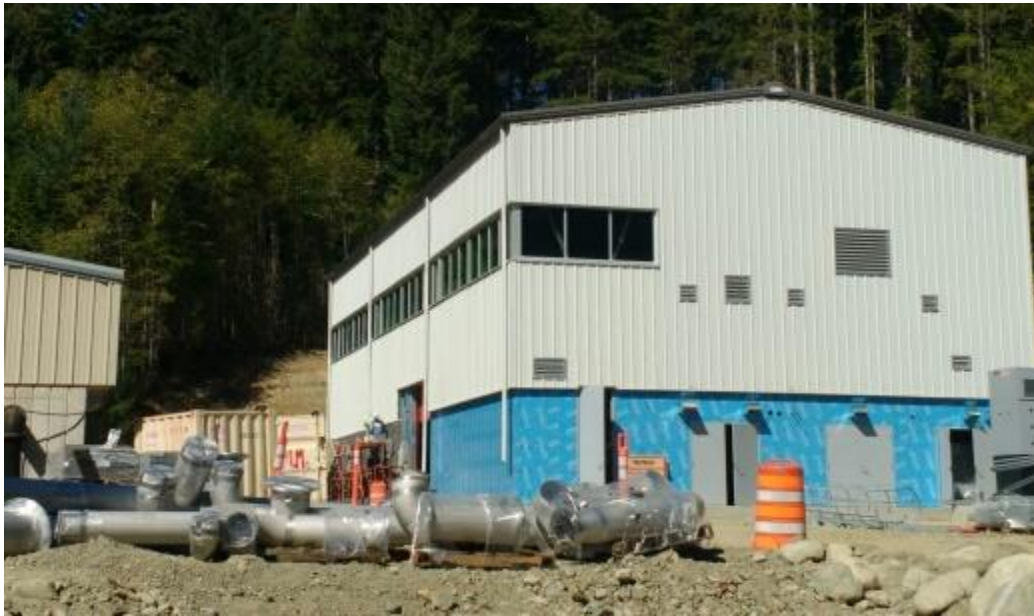
Figure 18 Water Treatment Facility on Indian Road
